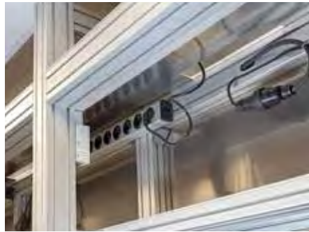
Cable routing from the roof to the workplaces.
