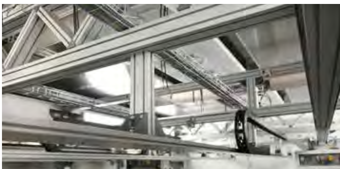
Linear system in the ceiling area for handling the weight chains in the chamber.
